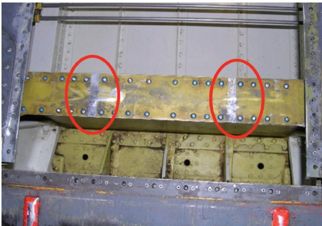
Figure 1: Chafing damage to the floor structure.
